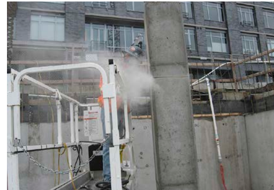
Photo 1: Rework is often rushed and not properly planned, which can put trade workers at risk. In this photo, mispoured concrete has placed a worker at height and exposed to silica dusts.
